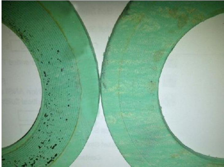
Figure 51: Uneven Gasket Compression
